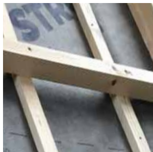
rear ventilation opened
